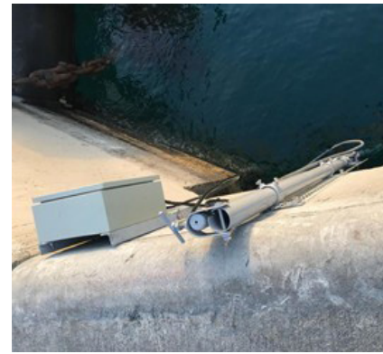
Tide Sensor installed at Port Jetty
