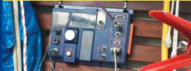
Aanderaa SmartGuard housed in the forward sail locker.
